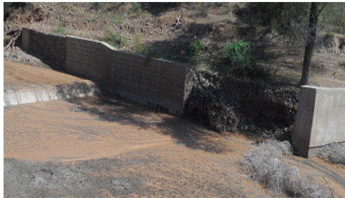
Figure 4-6 Destroyed gabion at Oneya diversion head work, 2013
