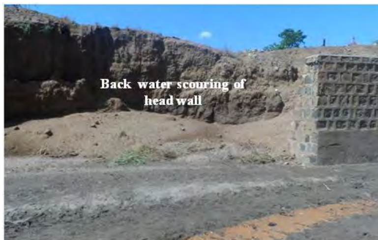
Figure 4-20 Back scouring of the head wall at Oneya diversion structure, 2013
