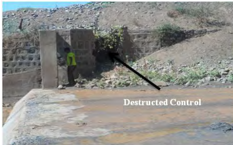
Figure 4-19 The destructed gate and high accumulation of sediment on the diversion weir at Oneya diversion structure
